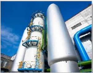
Industrial Air Quality Engineering expertise
